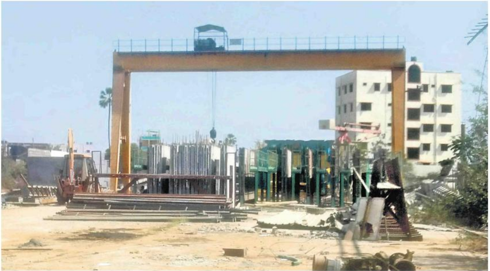
COST-EFFICIENT: Once the designs are ready, the walls are cast at the site (in-situ) and assembled using cranes.
