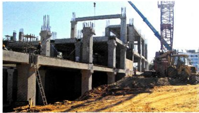
Precast technology has been adopted for faster execution and achieve quality construction with less wastage.
