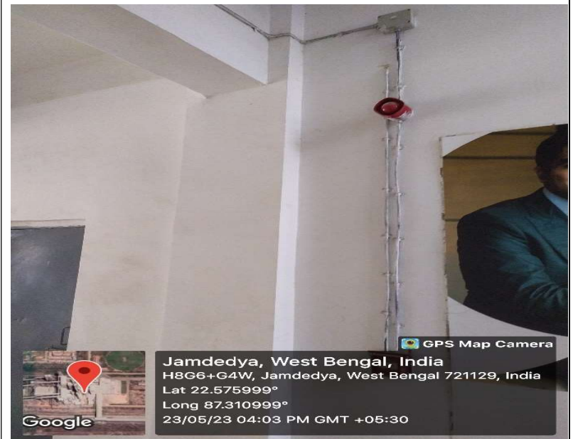
Fire Alarm (Photograph-XXXI)
