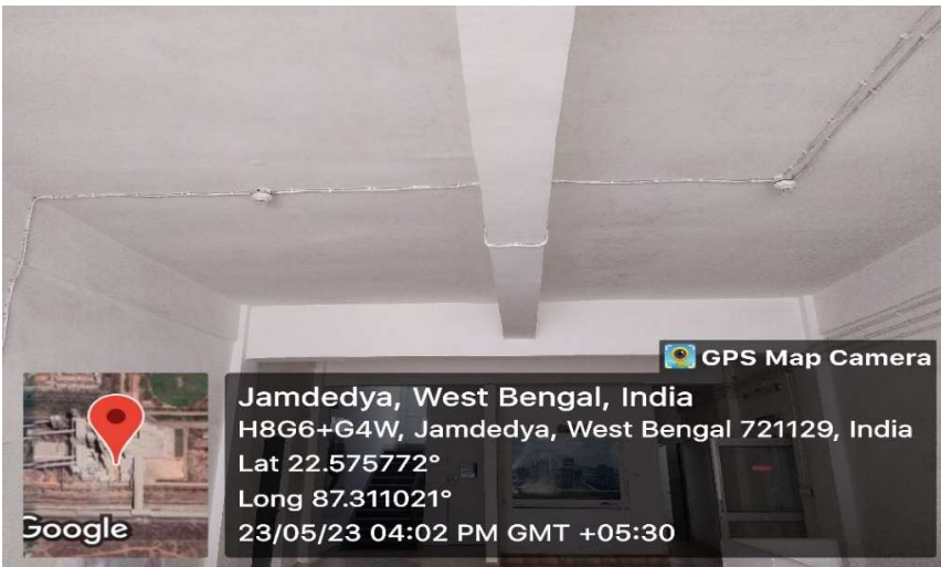
Smoke Detection Sensor (Photograph-XXXII)
