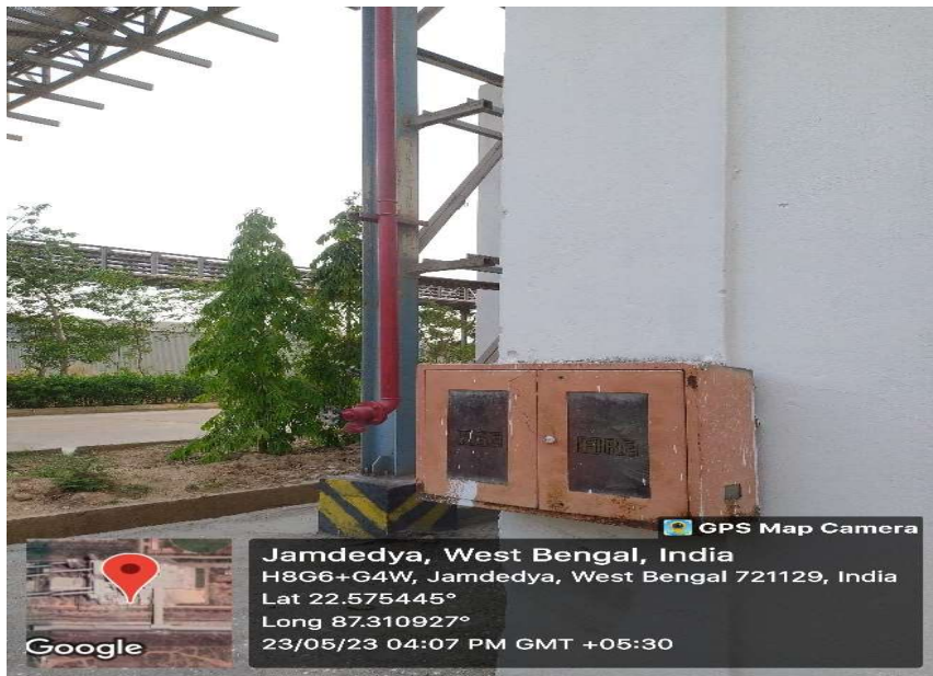
Fire Fighting System (Photograph-XXX)
