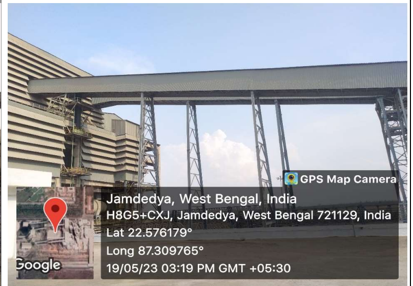
Covered belt conveyors (Photograph - IX)
