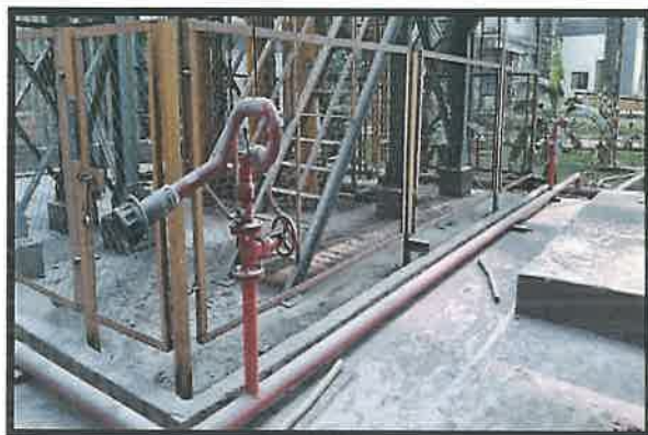
Photo – 12: Firefighting arrangements
