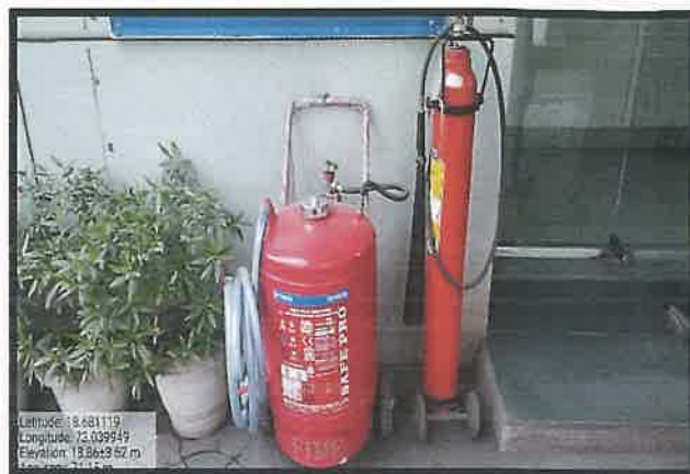
Photo – 13: Firefighting arrangements
