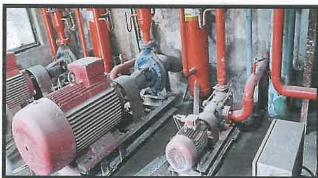
Photo – 14: Firefighting arrangements
