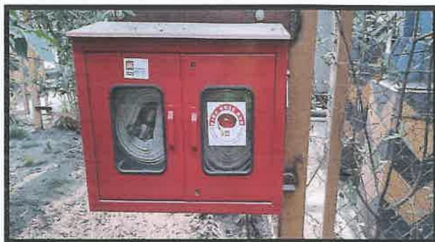
Photo – 15: Firefighting arrangements
