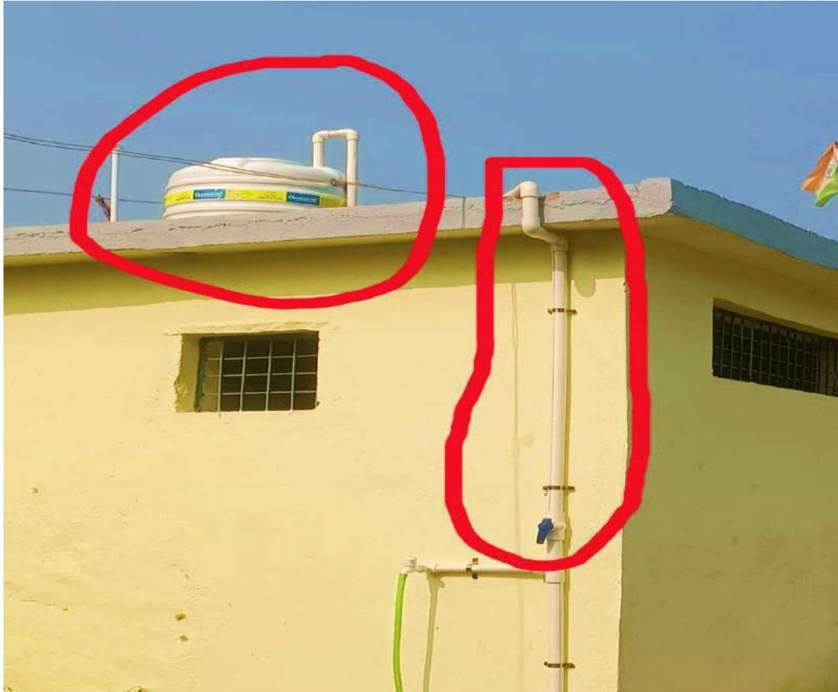
Water overhead tank connection fitting for continue water supply in School premises –Middle School on 22 nd Nov-2024
