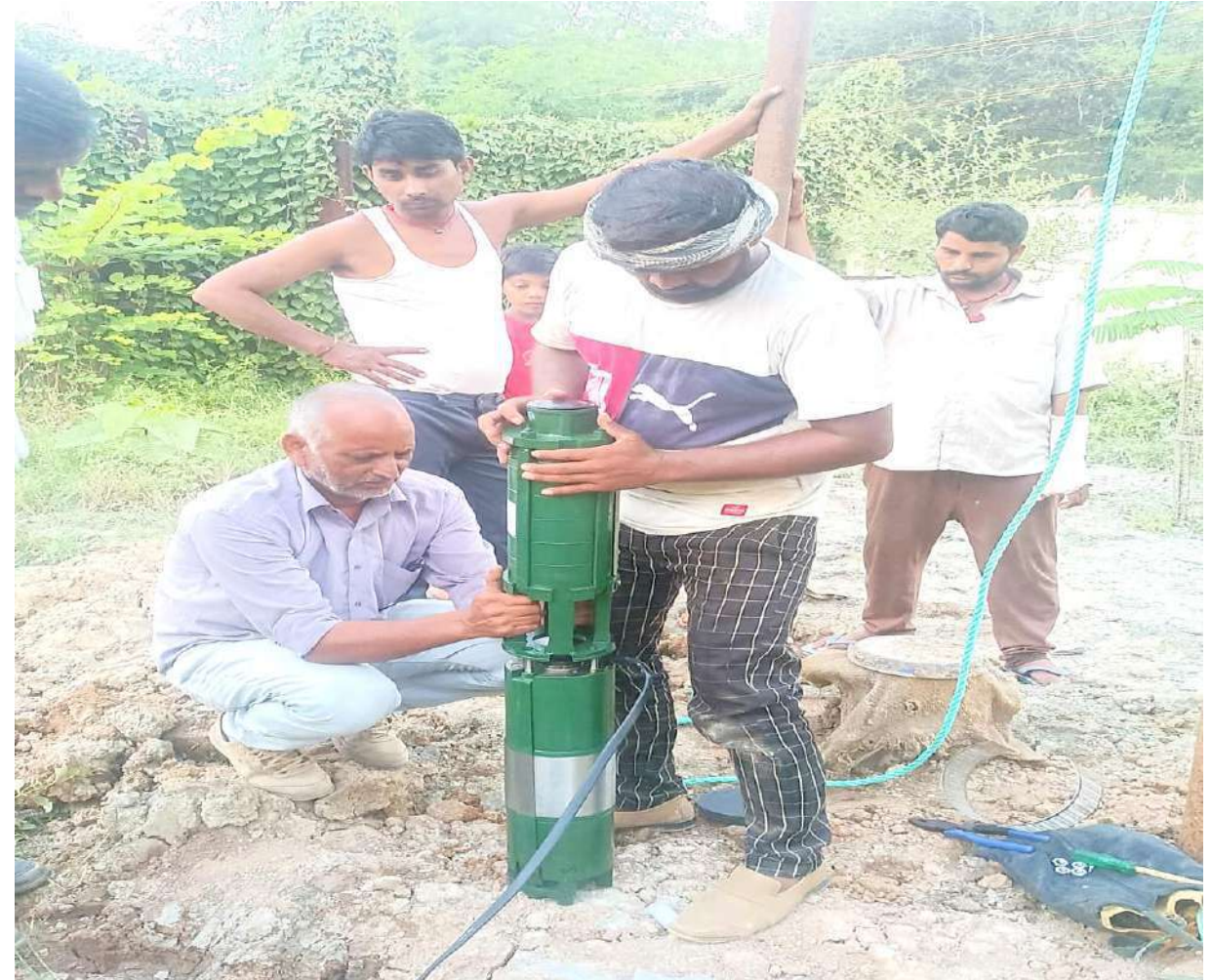
Photographs during fitting the Submersible pump at Kolkarhiya Middle School on 26 th Oct, 24
