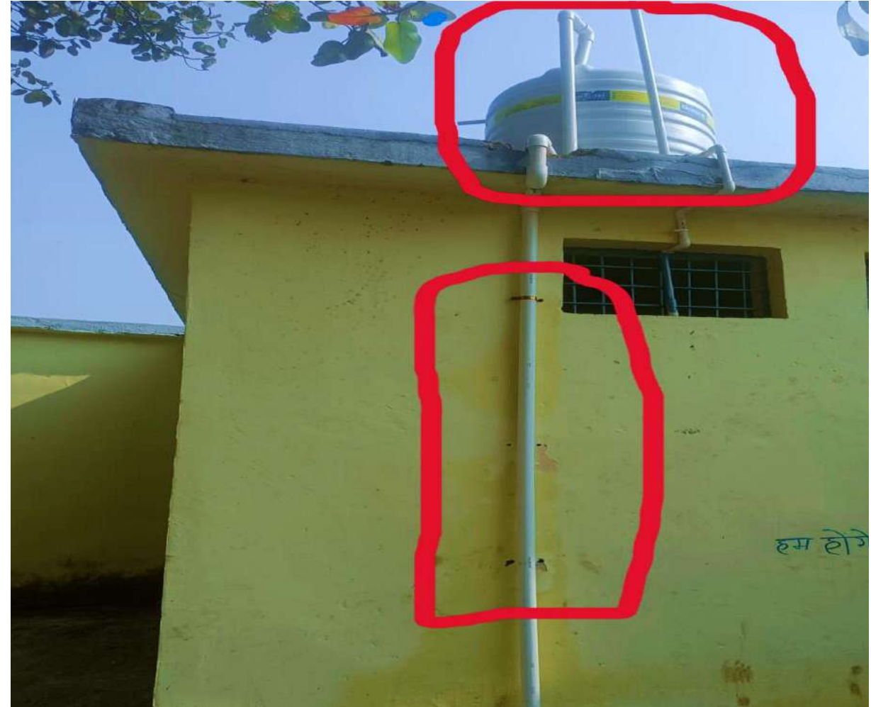
Water overhead tank connection fitting for continue water supply in School premises –Primary School on 22 nd Nov-2024
