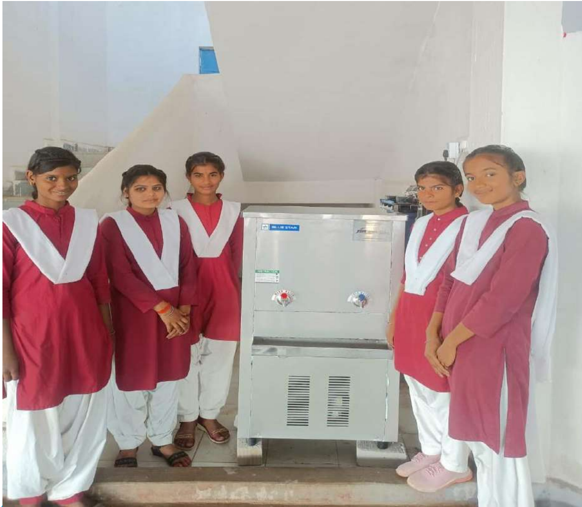
Water Cooler installation at Gaisabad Higher Secondary School, benefited around 490 plus students
