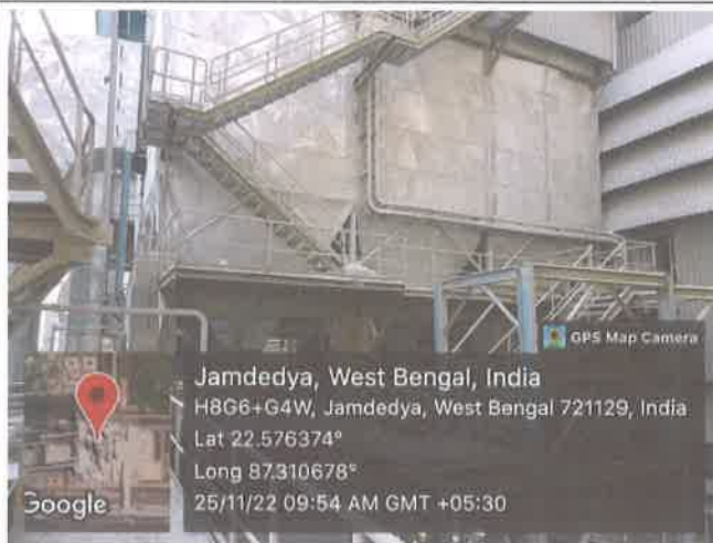
BAG HOUSE ATTACHED TO GRINDING UNIT : (Photograph-2)
