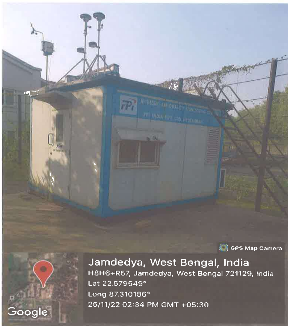
AMBIENT AIR QUALITY MONITORING STATION (Photograph- 04)
