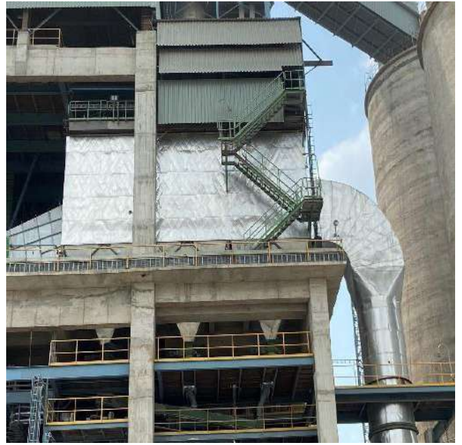
Main baghouse of the Roller Press
