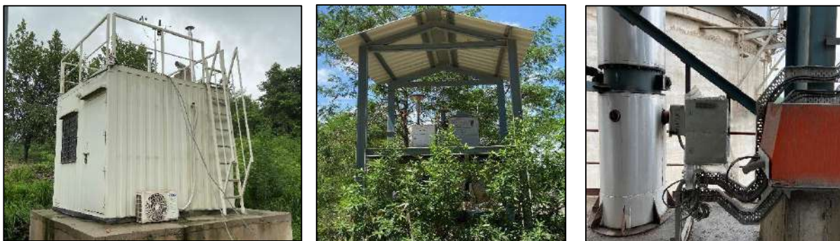
Continuous Ambient Air Quality Monitoring System
