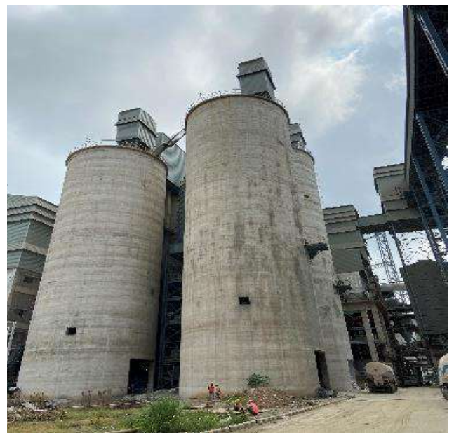
Closed Silo installed for Final Products
